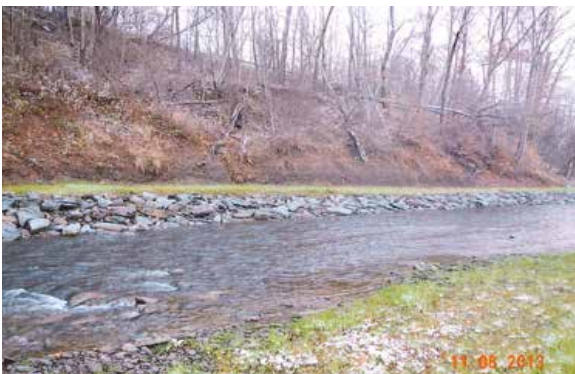
Looking upstream after construction at rock riprap toe with bench Thomson Cross Road at the top of the bank.
