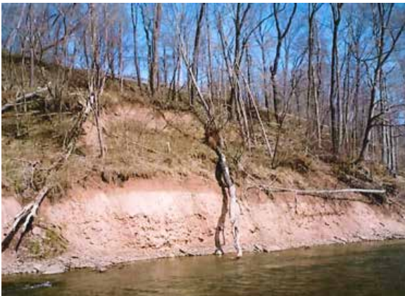
Looking upstream at the eroding bank with Thomson Cross Road at the top of the bank.
